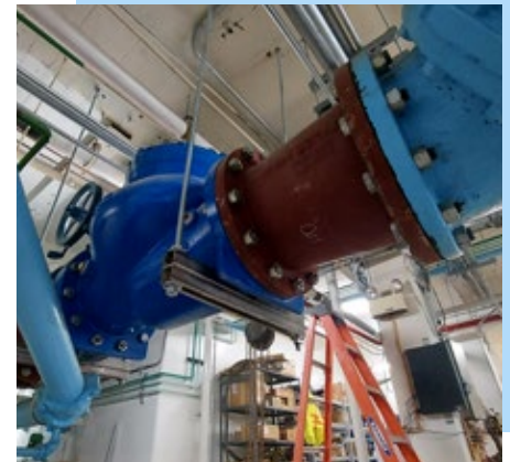
This pressure reducing valve (PRV) now safely controls the water pressure used during a filter backwash. This system backs up the two new backwash pumps.
