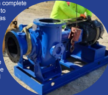
This is one of two new backwash pumps in service as of June 2021.
