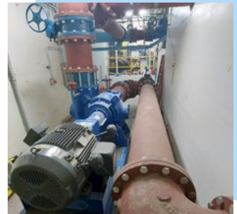
One of the two backwash pumps installed ready for paint.
