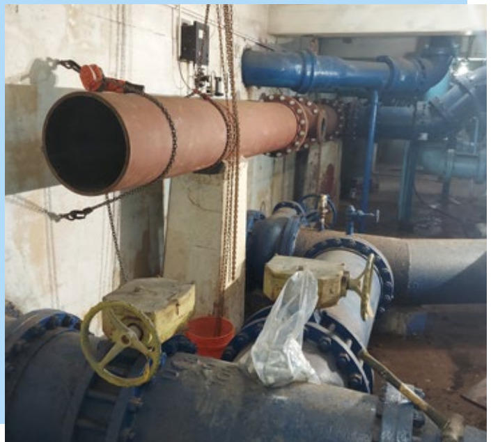
New 16" piping being installed in the subbasement of the Plant replacing a 80+ year old pipe that was ready to burst.
