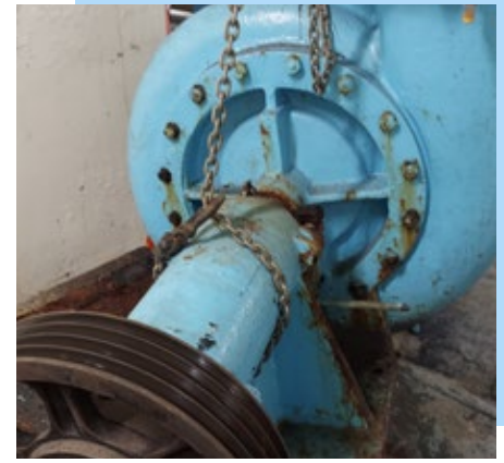
This original backwash pump was in service for 80+ years. There was no backup pump or usable backwash method if this failed.
