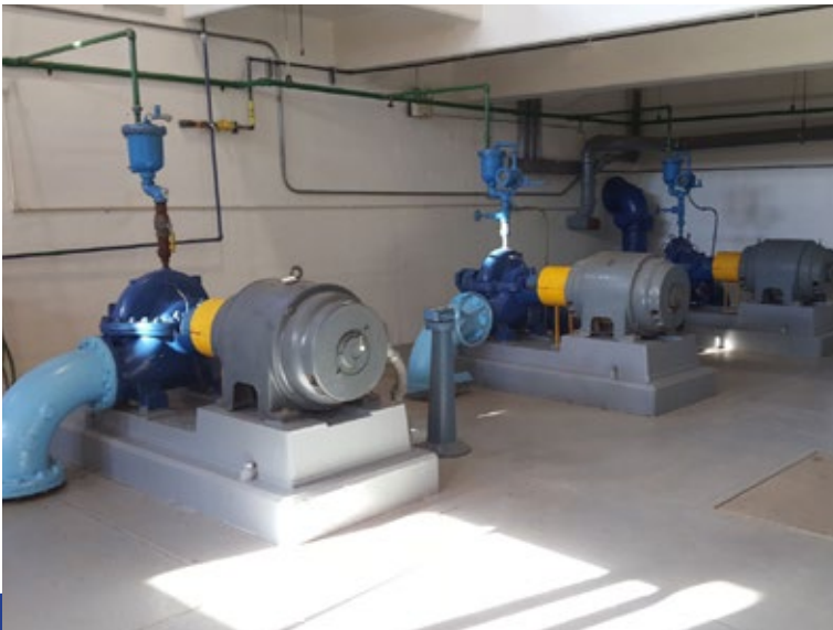
High Service Pumps 1, 2 and 3 shown above, pump 1 (furthest away) is being rebuilt.
