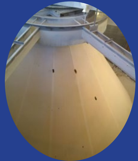
One of two Clarifiers at the Water Filtration Plant, the main bearing which required replacement, is located at the top of the cone which is 30 ft. deep.
