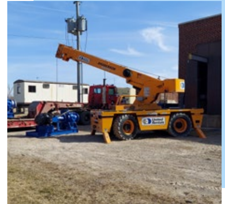
One of two new backwash pumps that were being unloaded for installation.
