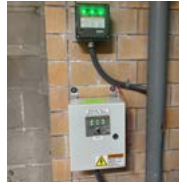
One of two surge protection installations to protect WTP backwash VFD's
