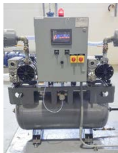
New vacuum pump system for WTP high-service pumps
