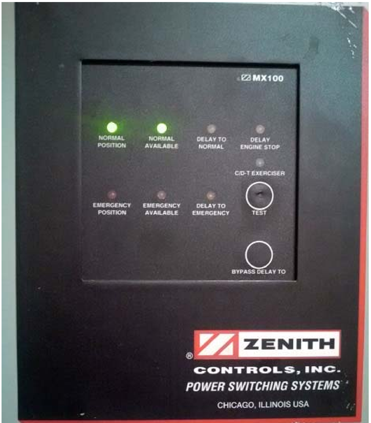
Existing Automatic Transfer Switch Control Panel
