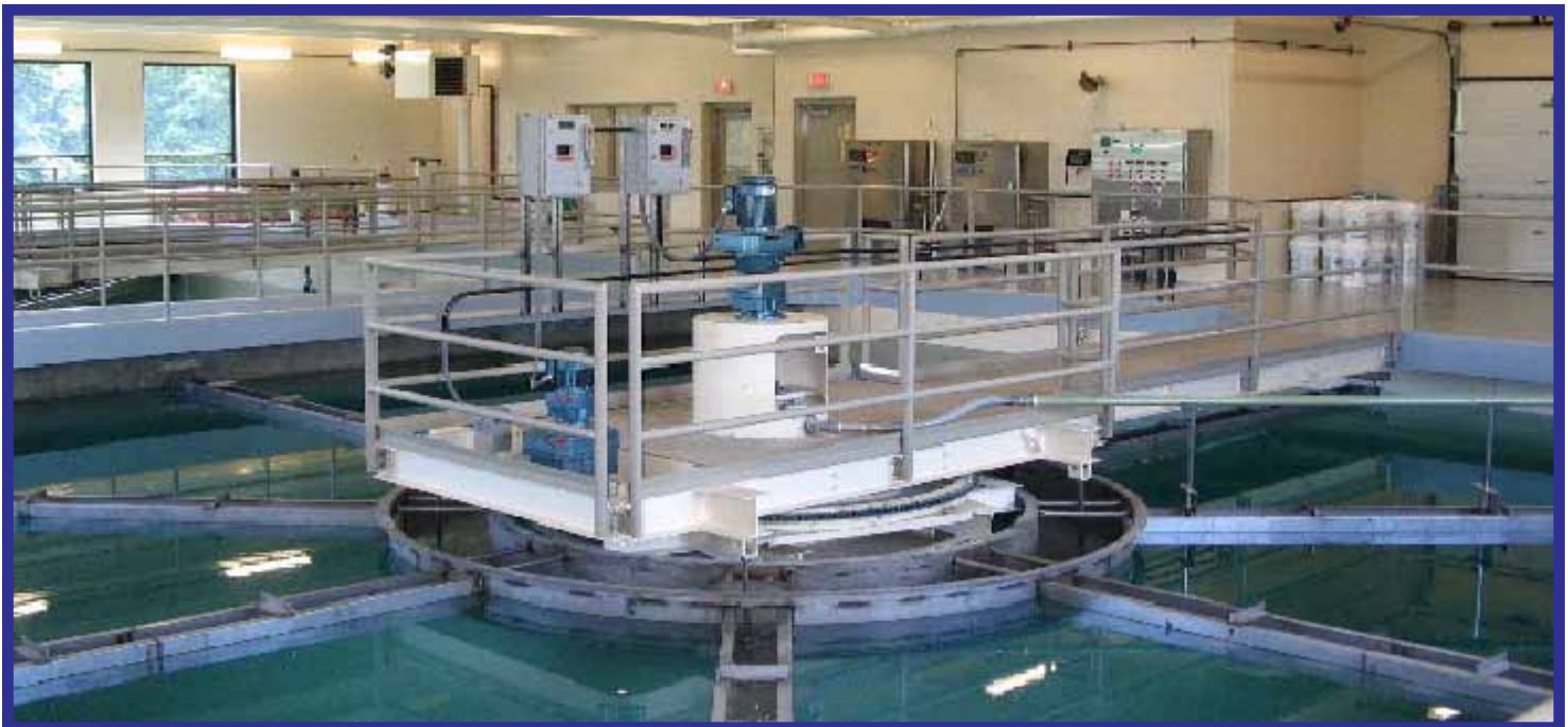
New lime softening clarifiers, part of a $4.8 million water treatment plant improvement project, were fully operational in April, 2004.
